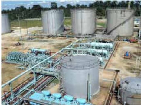
Flow Station showing Tank Farms
