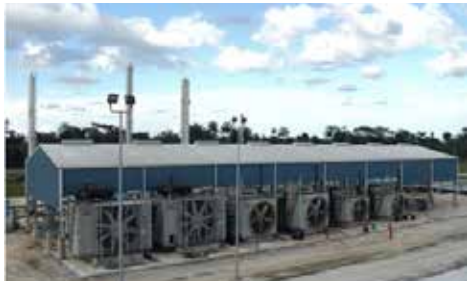
Gas Plant Showing Compressors- Side View
